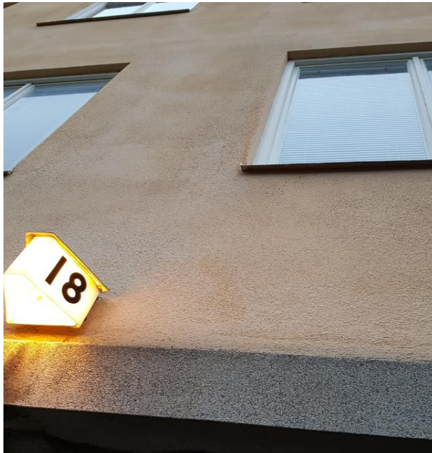
Figur 2. Fasad i ok skick.
